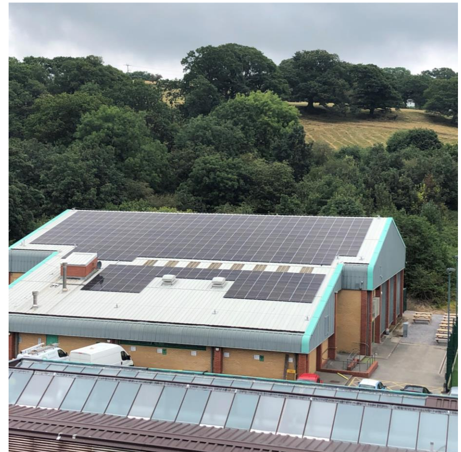
Figure 1.1.1: Solar panels at Ysgol Dinas Bran, Llangollen
